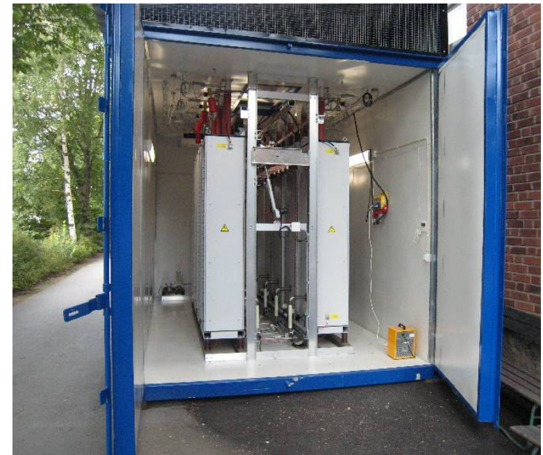
Picture of the new Li-ion battery after testing, October 2008
